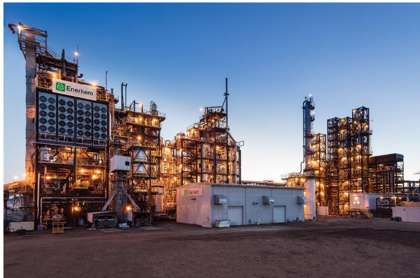
Enerkem Alberta Biofuels waste-to-biofuels and chemicals facility in Edmonton
